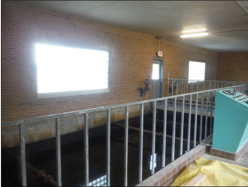
Figure 42. View of the interior basins, second story of the office and treatment building at the T. J. Ellison Water Treatment Facility.
