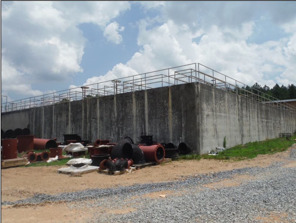
Figure 36. View of the office and treatment building at the T. J. Ellison Water Treatment Facility, basins on rear elevation, facing southeast
