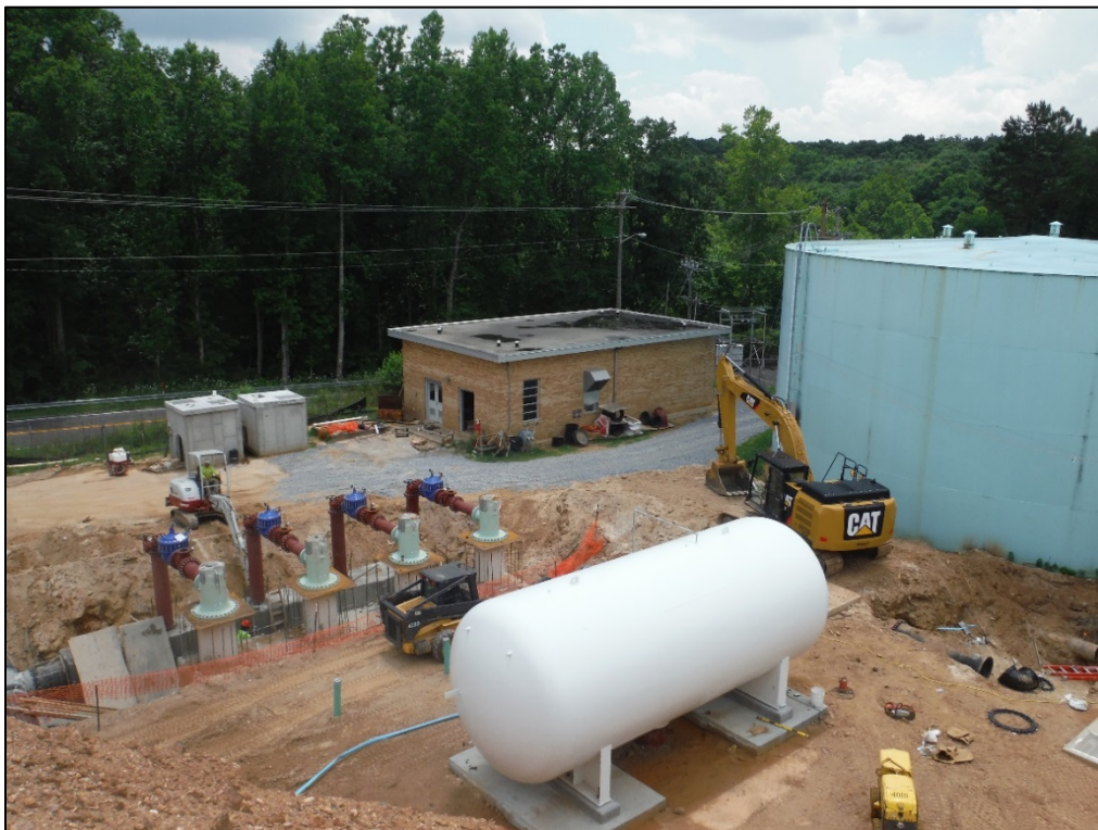
Figure 54. View of the pump building and new pumps at the T. J. Ellison Water Treatment Facility, facing southwest.
