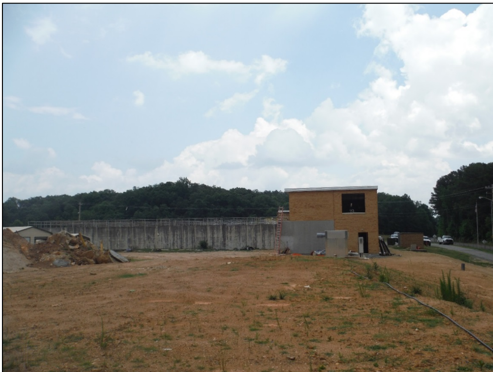
Figure 34. View of the office and treatment building at the T. J. Ellison Water Treatment Facility, west elevation facing east.
