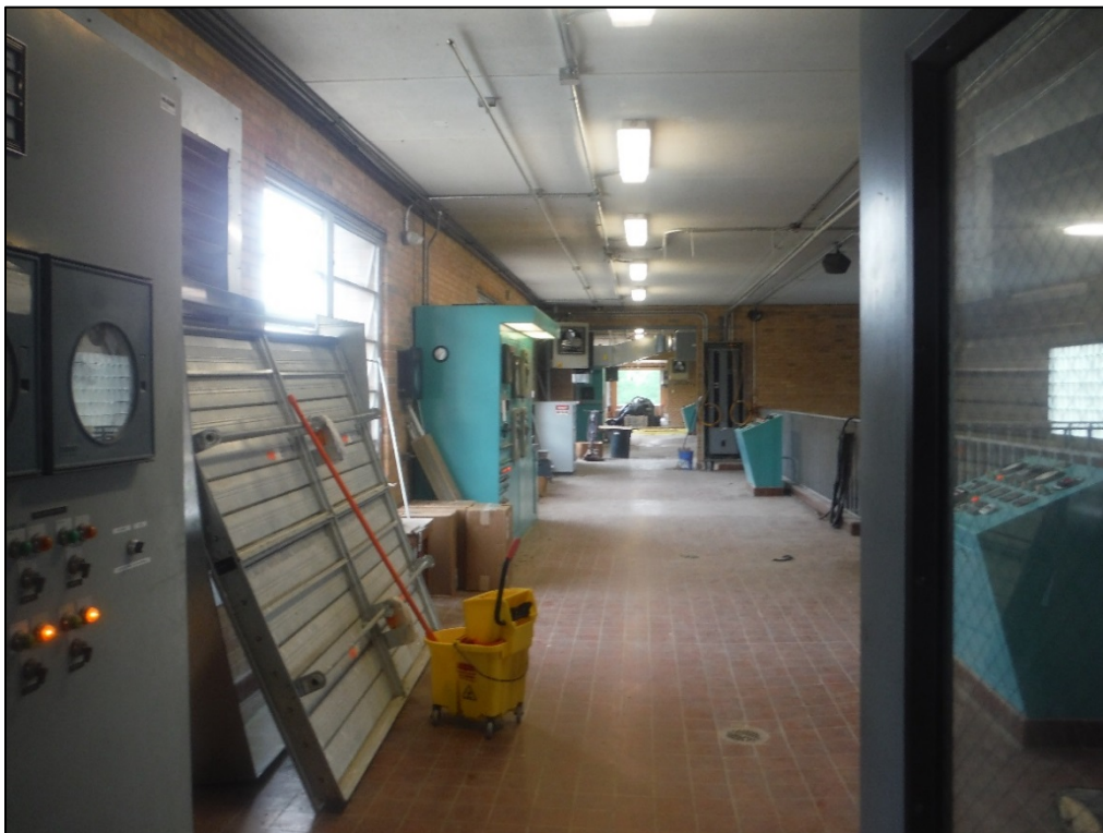
Figure 41. View of the interior corridor, second story of the office and treatment building at the T. J. Ellison Water Treatment Facility.
