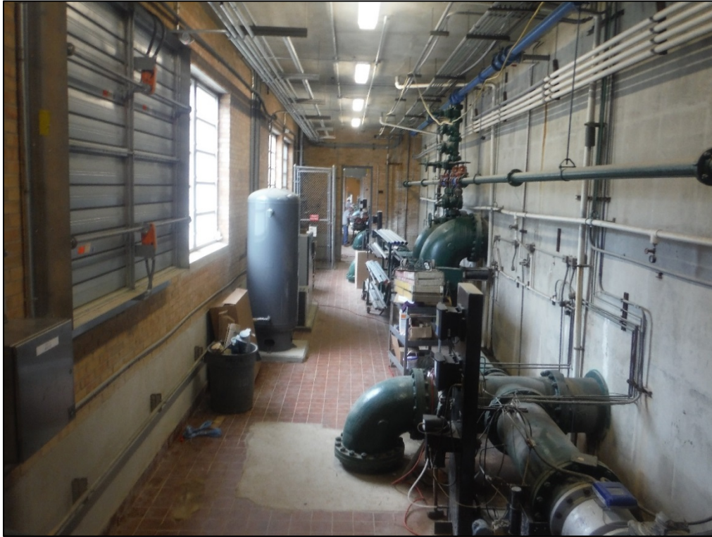
Figure 40. View of the interior corridor, first story of the office and treatment building at the T. J. Ellison Water Treatment Facility.
