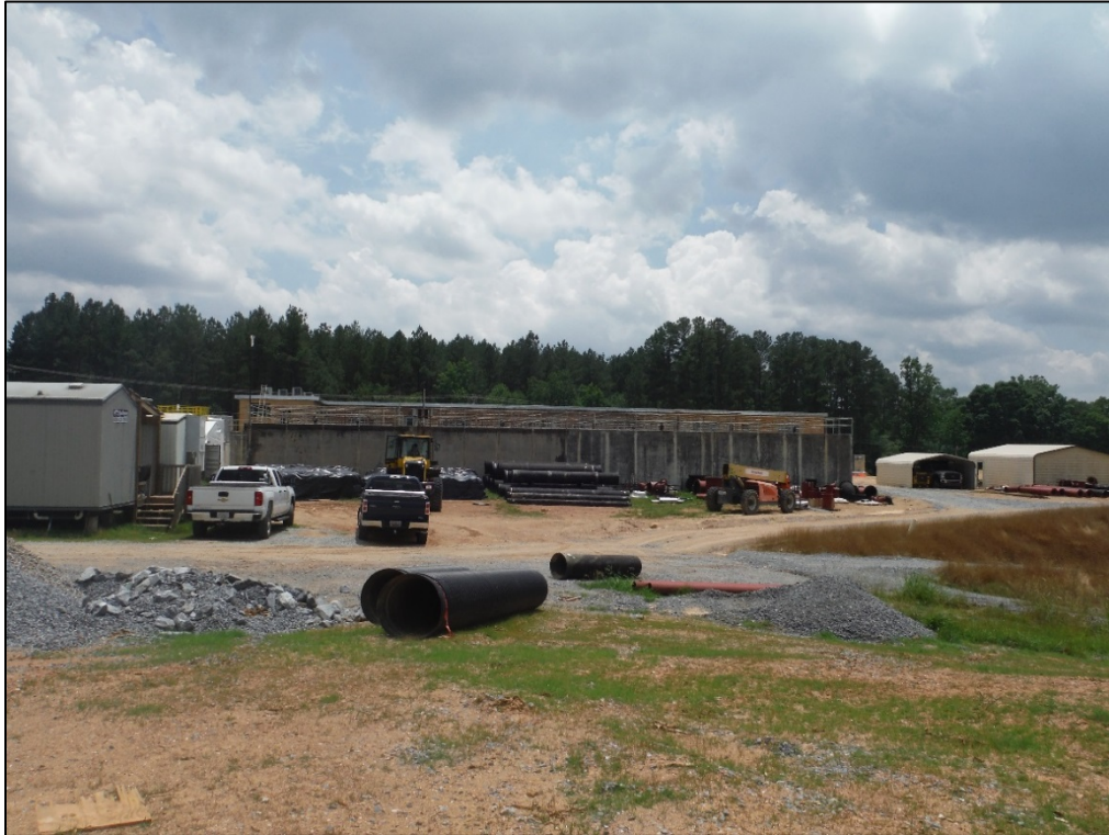
Figure 37. View of the office and treatment building at the T. J. Ellison Water Treatment Facility, rear elevation, and metal storage building and carport, facing south.
