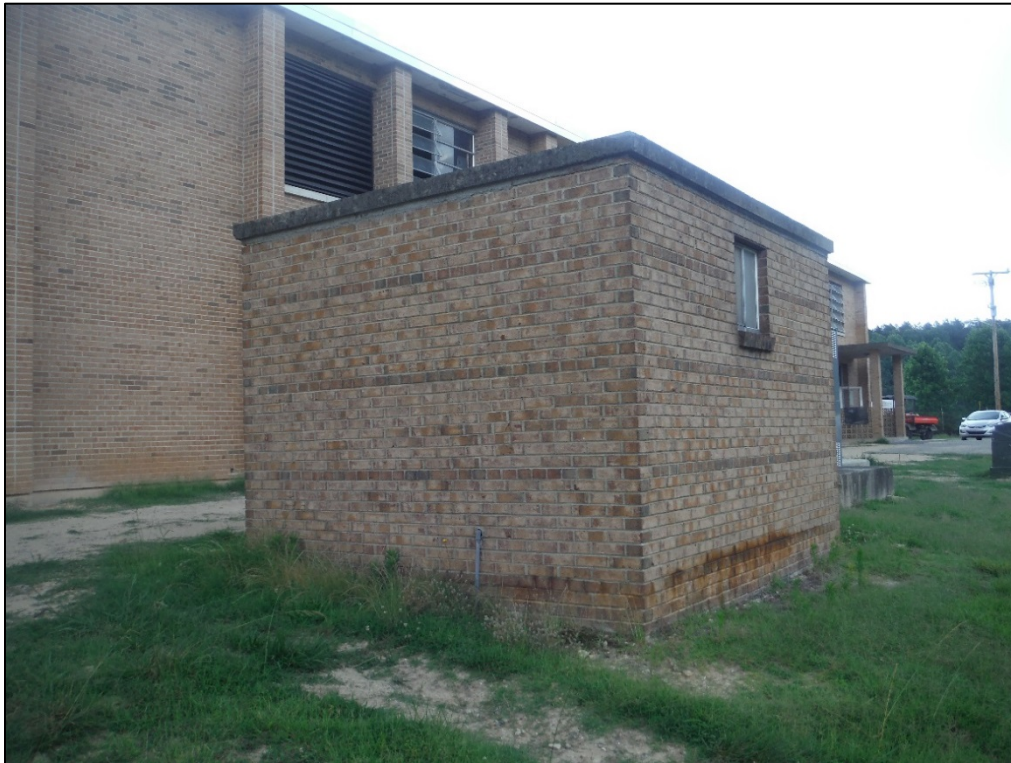
Figure 56. View of the electrical building at the T. J. Ellison Water Treatment Facility, facing northeast.
