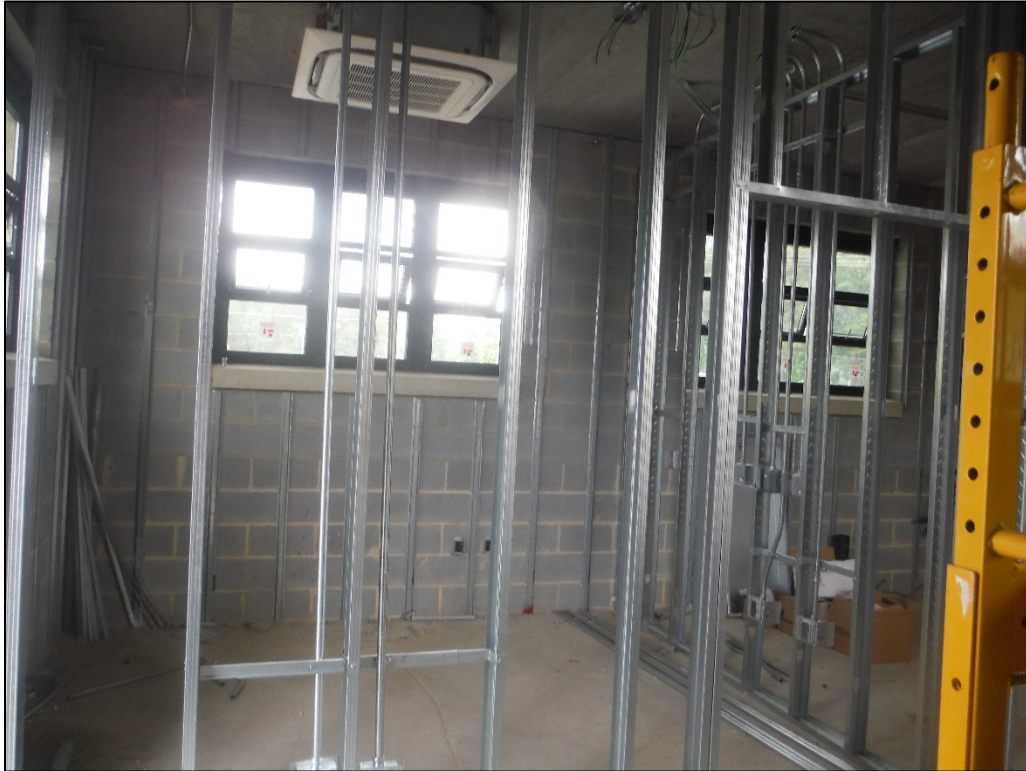
Figure 46. View of the new office/laboratory, under construction on the second story of the T. J. Ellison Water Treatment Facility.
