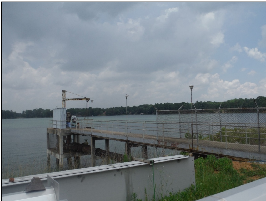
Figure 48. View of the raw water pumps at the T. J. Ellison Water Treatment Facility, facing north.
