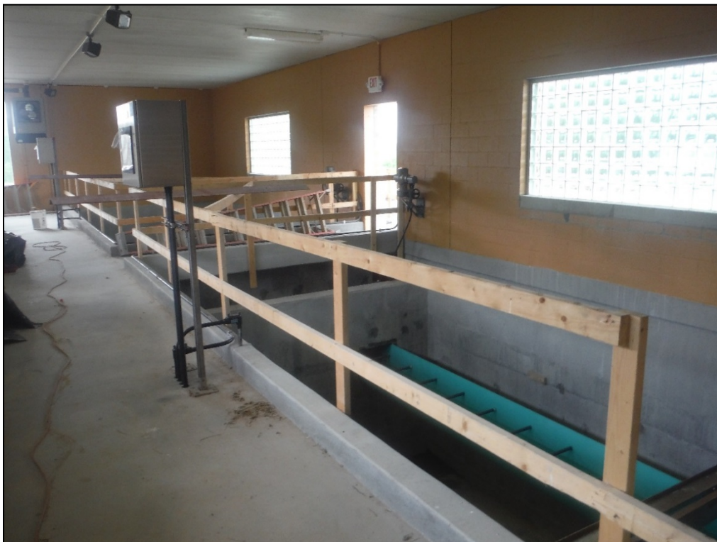
Figure 43. View of the interior basins, second story of the office and treatment building at the T. J. Ellison Water Treatment Facility.
