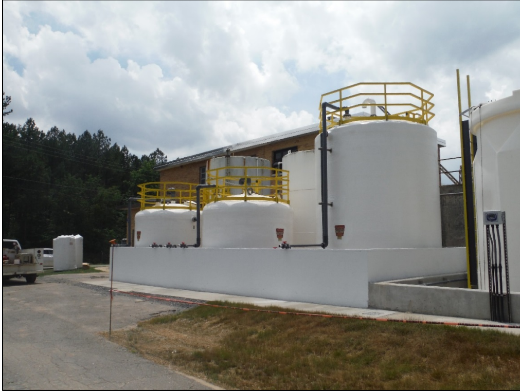
Figure 47. View of the modern plastic tanks at the T. J. Ellison Water Treatment Facility, facing southwest.
