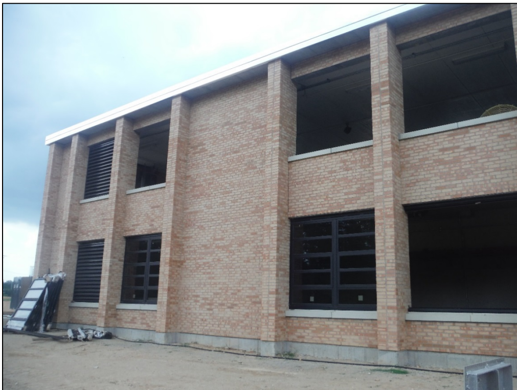
Figure 32. View of the office and treatment building at the T. J. Ellison Water Treatment Facility, facing northwest.
