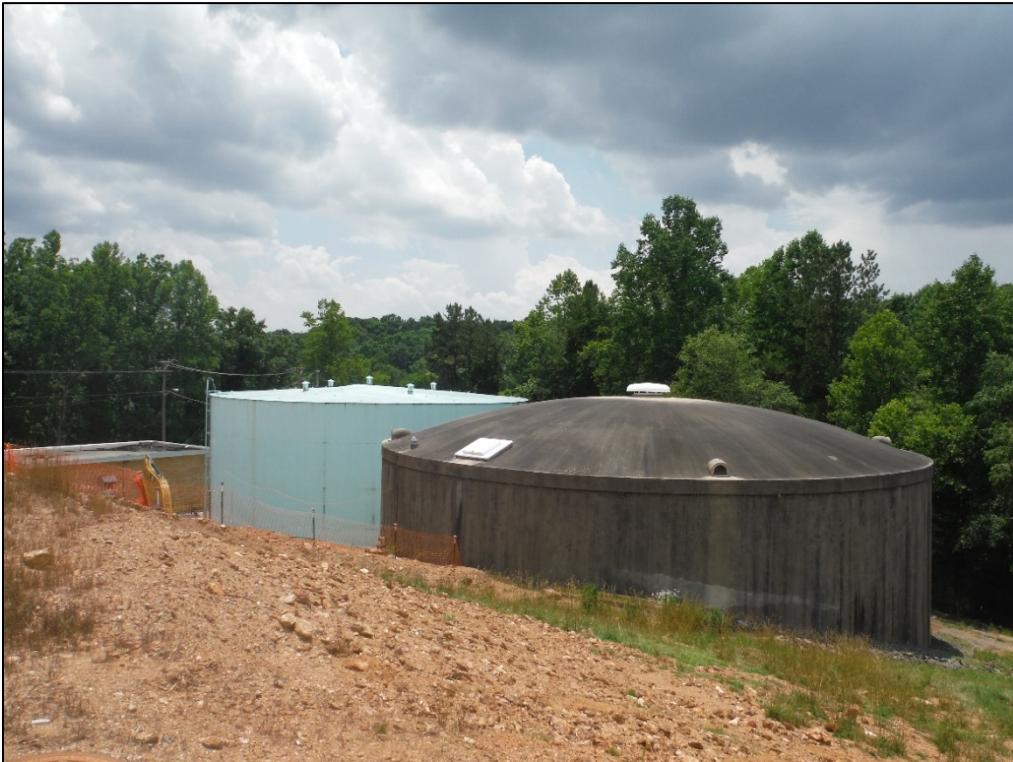
Figure 52. View of two holding tanks at the T. J. Ellison Water Treatment Facility, facing southwest.
