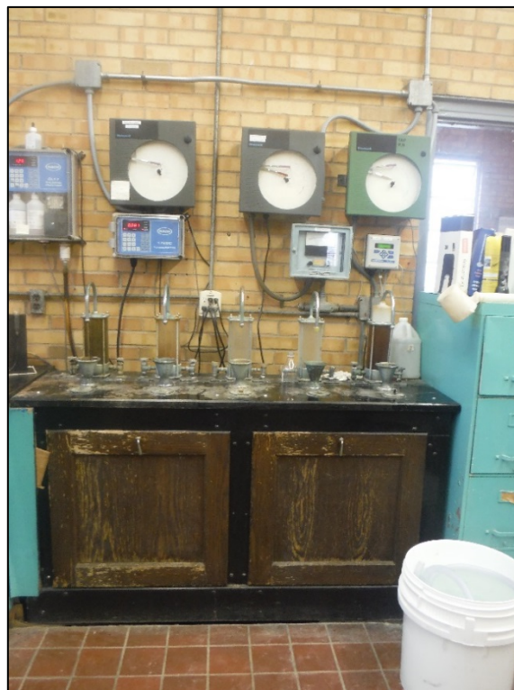
Figure 45. View of the office/laboratory/break room, second story of the T. J. Ellison Water Treatment Facility.
